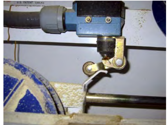
Photo #4 - Safety Switch (Roller Switch for Drive)
