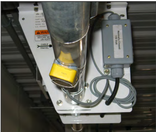
LOOKING AT MOTORIZED HOPPER
