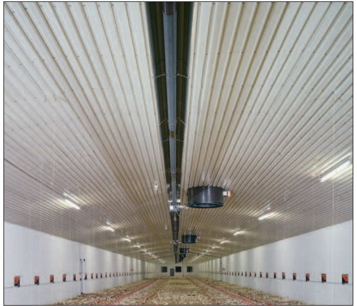
Implementation of infrared heaters in a broiler house
