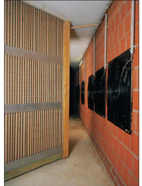
Rear side of the filter, ventilators suck the air through the wall
