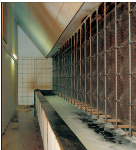
Nozzle groups spray water onto the front of the filter bank so that dust cannot cling to the filter bank. The individual filter chamber doors
